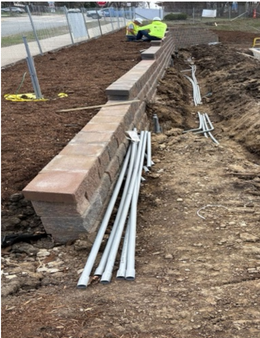
Electrical underground at retaining wall
